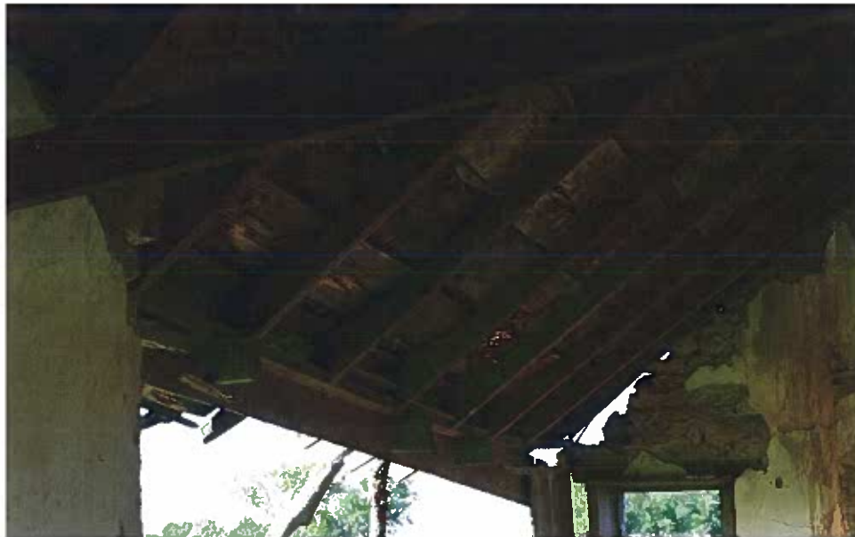
PHOTO 4: LOCALIZED PUNCTURE IN ROOF AT CENTER OF PICTURE
