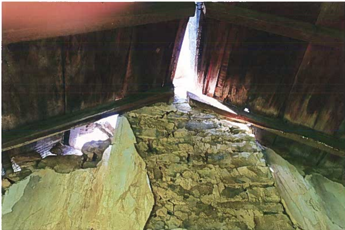
PHOTO 10: RAFTER BEAM STARTING TO OPENING UP AT THE ROOF RIDGE ON WEST END.
