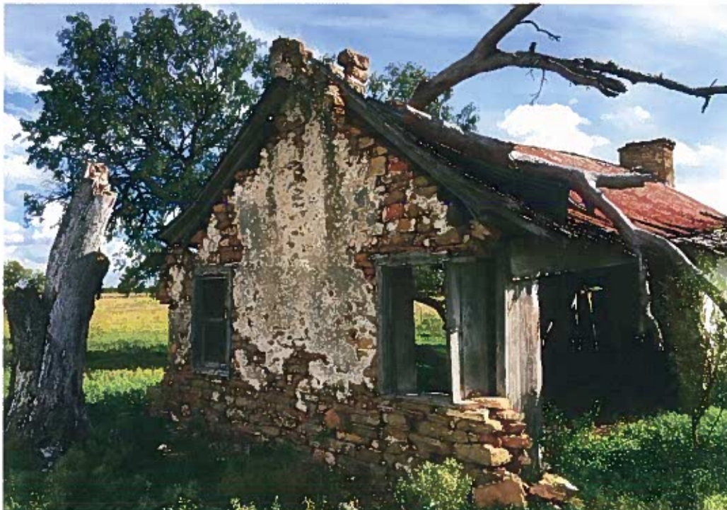
PHOTO 3: TREE ON ROOF AND EXCESSIVE DEFLECTIONS AND DISTRESS
