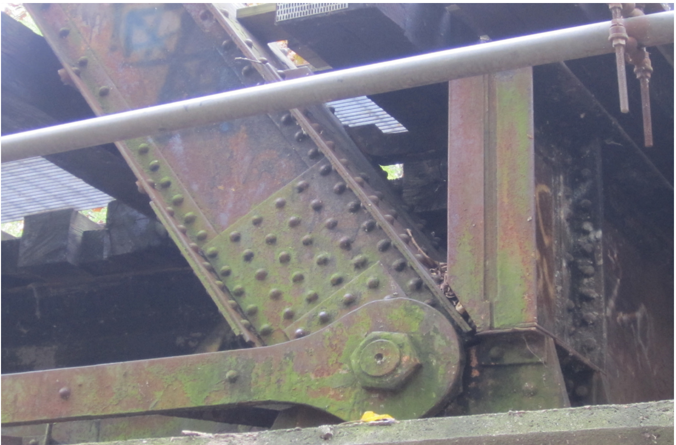
Bridge MP 40.19 Photo 11 - Looking Northeast at West Elevation Lower Chord & End Post Connection Deterioration
