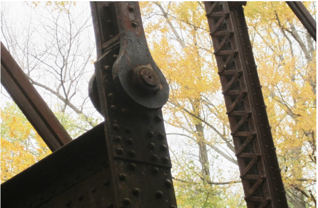
Bridge MP 40.19 Photo 10 - Looking Northwest at Bridge Deterioration at Pinned Connection
