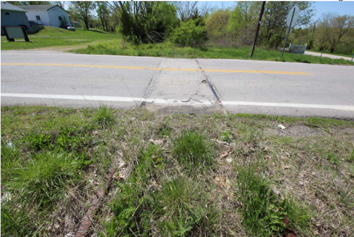
Photo 11: Paved Over Track at Hwy CC, between Mile Markers 74.00 and 75.00, Facing West
