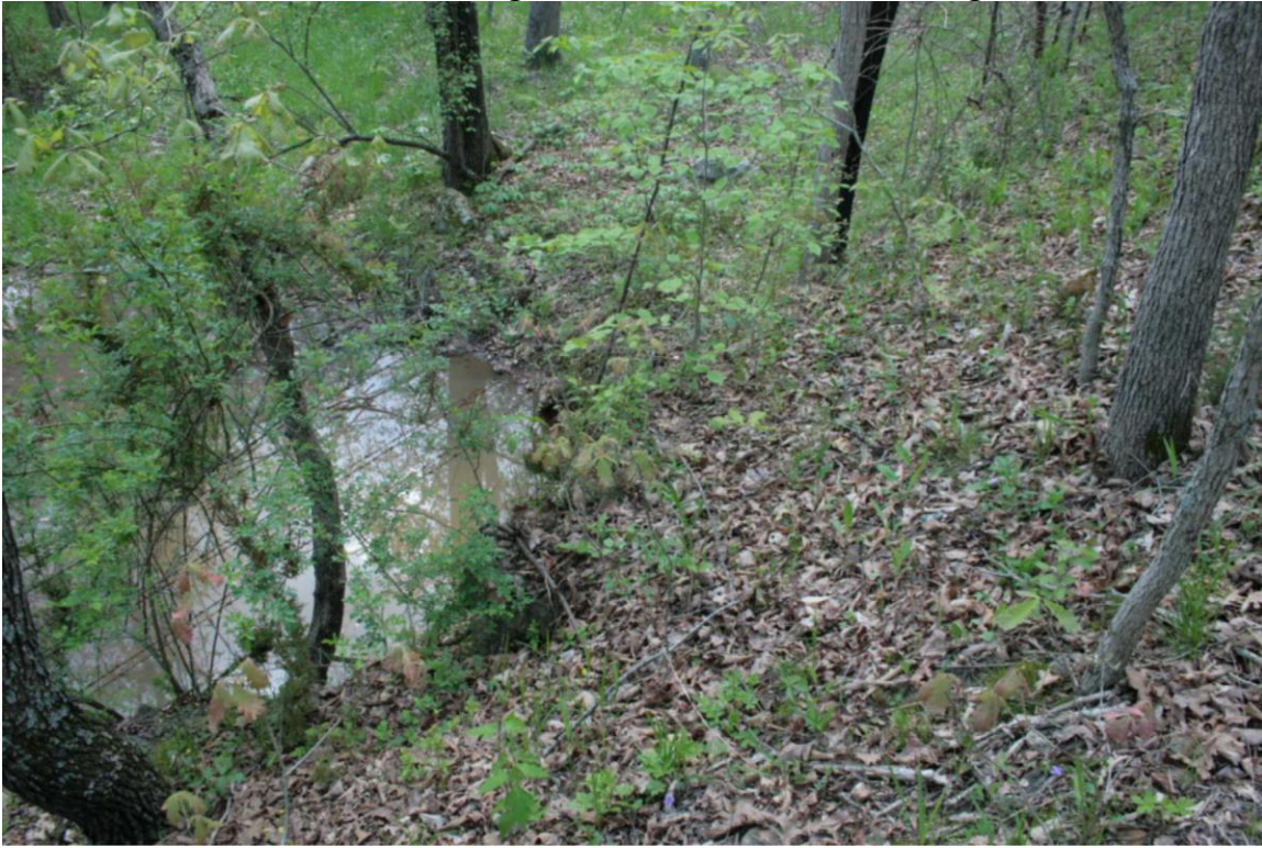
Photo 7: Fence Obstructing Access to Culvert 86.00, Facing Southwest
