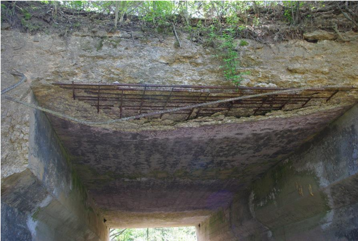
Photo 50: Culvert 88.92, Showing Partially Deteriorated Roof, Facing South
