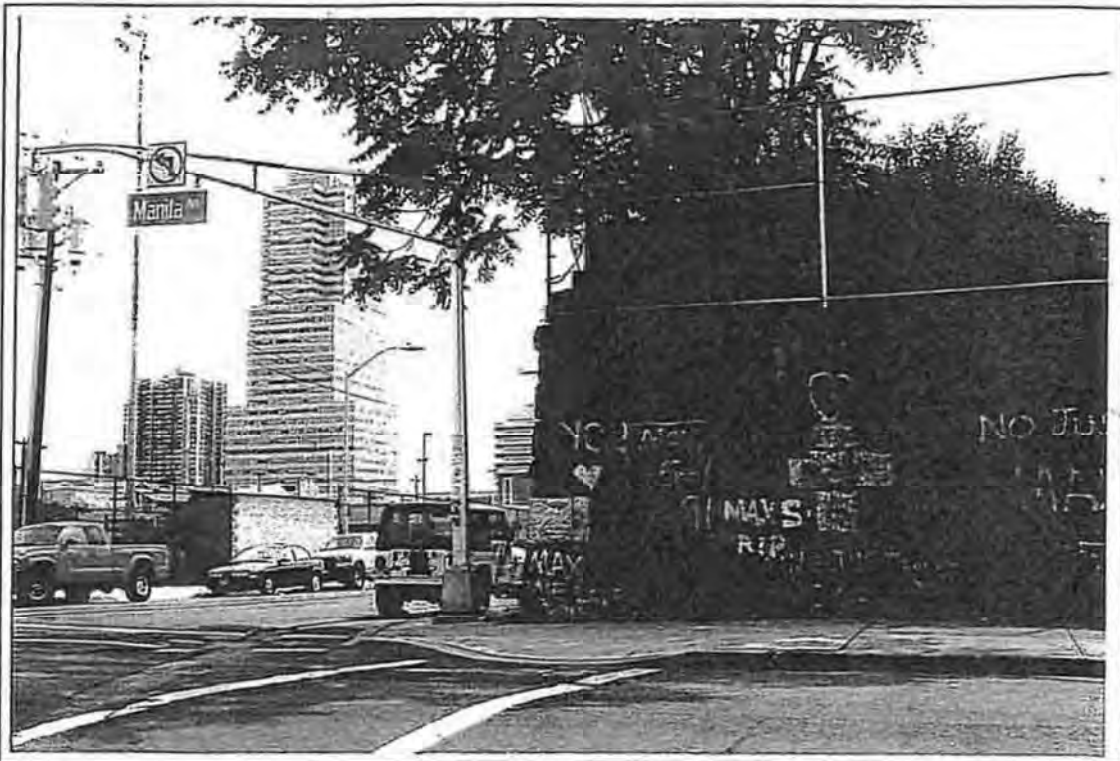
PLATE 5: Sections of Embankment are Deteriorating from Intrusive Vegetation and Marred with Graffiti
