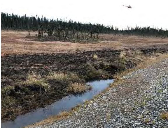
Photo 9. Localized Ponding at Uplift Area
