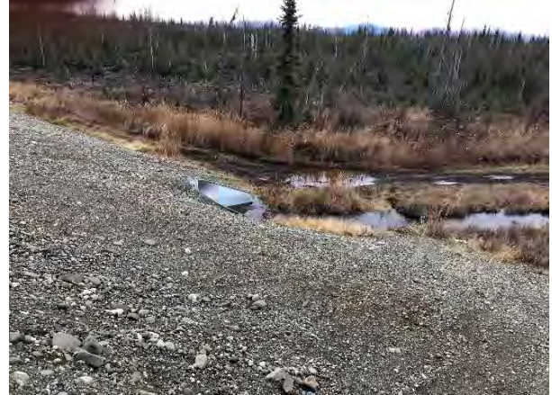
Photo 10. Evidence of ATV Use Adjacent to Culvert
