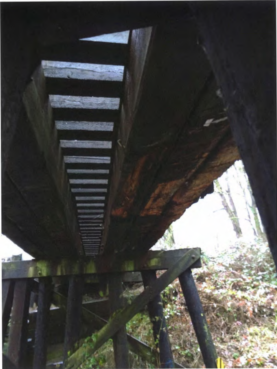
Span 2 West Stringer Damage and Timber Decay Looking South
