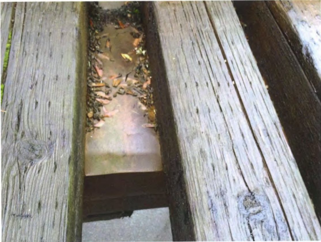
Top of West Inside Stringer Impact Damage at Bottom Looking West
