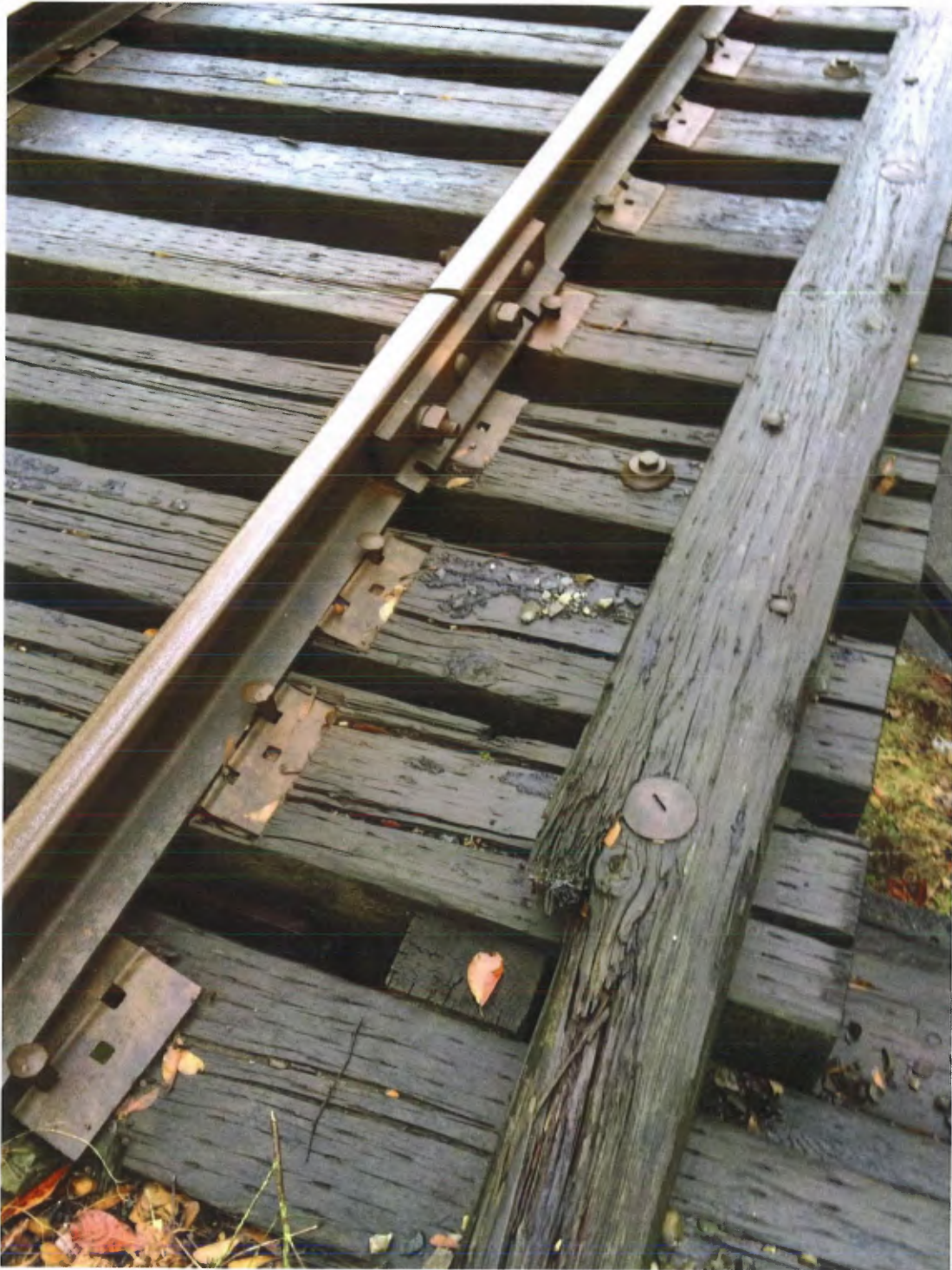
Tie Deterioration at North Span near Abutment
