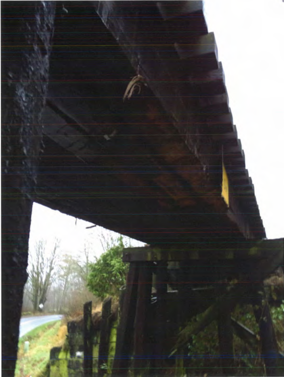
Span 2 West Stringer Impact Damage Looking Southeast
