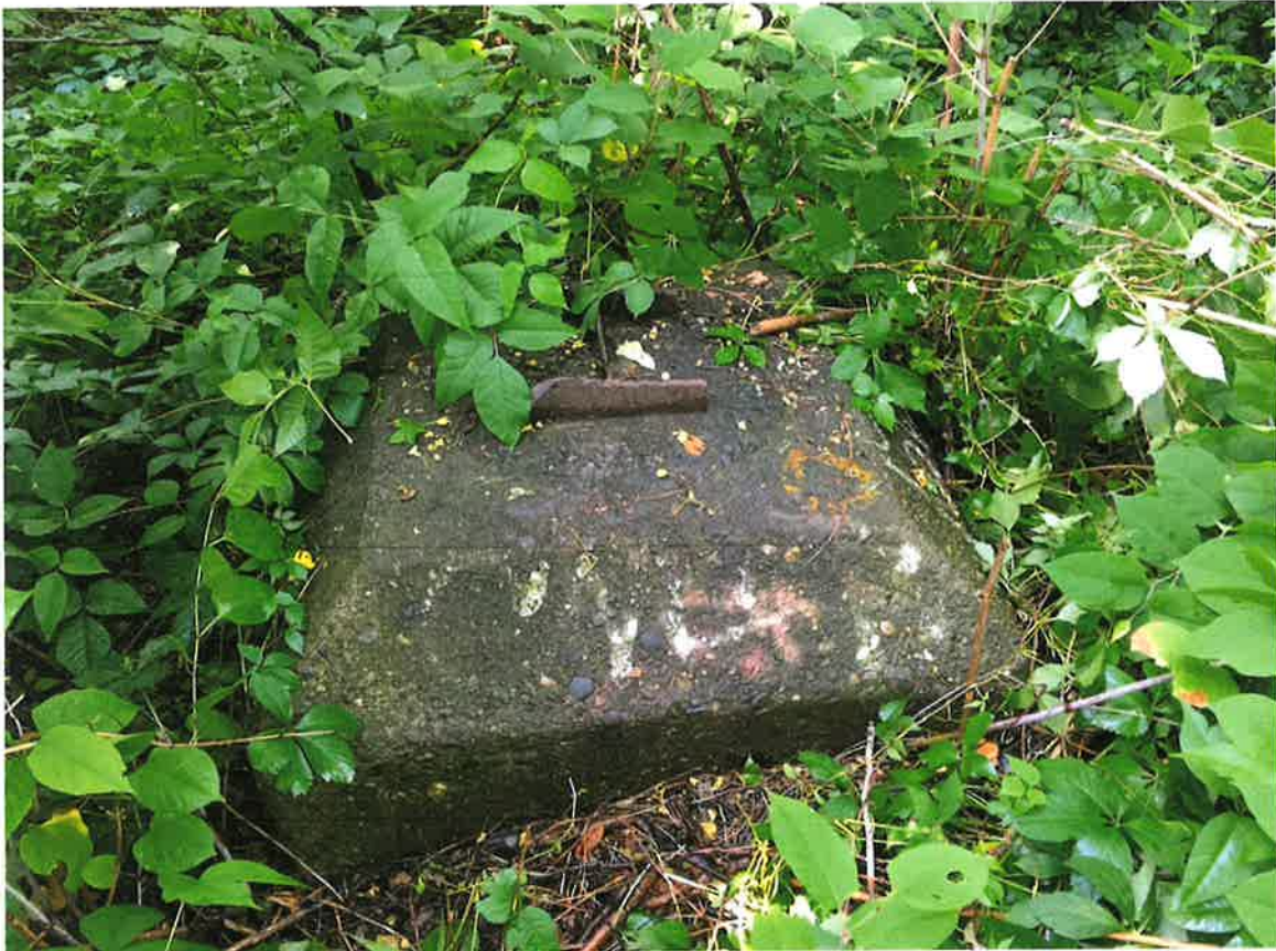
Photo 2. The matching south side catenary pole base.
