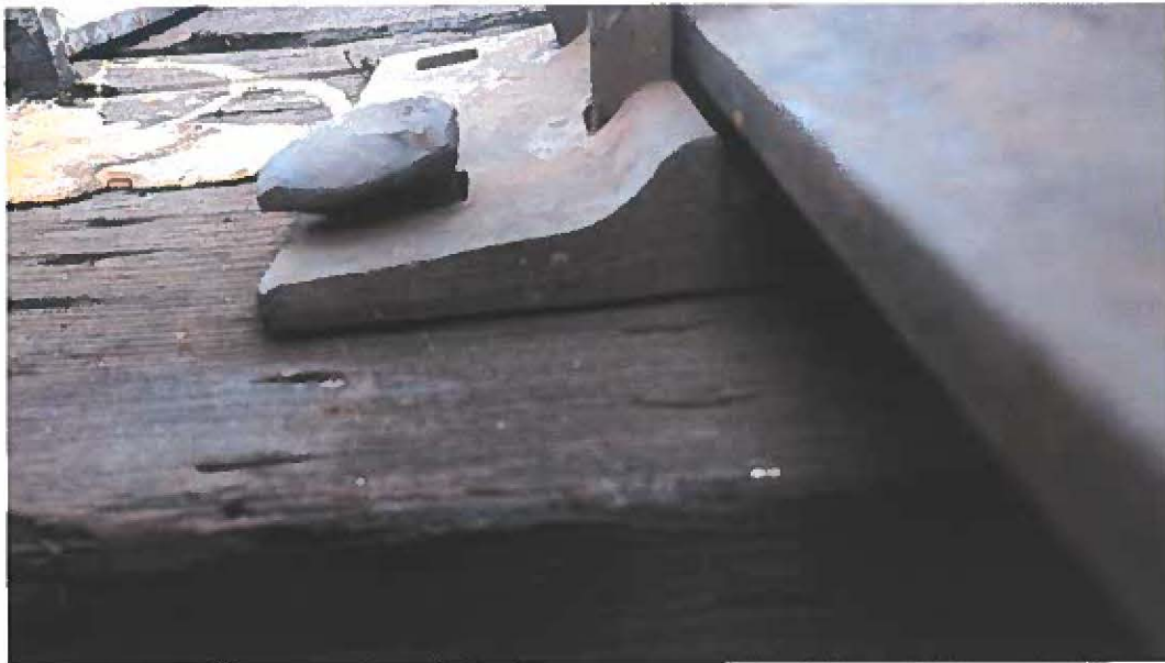
Picture 4 showing an existing tie that is next to a new tie. Although this may take some load of the rail, it is not taking the full designed load.
