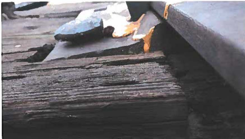
Picture 5 showing the Load Bearing Defect found on the bridge.
