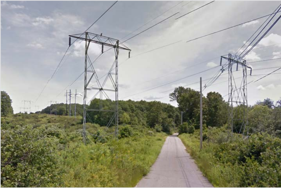
Power transmission lines at Cross Street in Millbury just North of where the bikepath and street will join.
