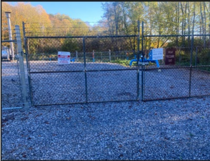
Natural Gas Station located below the old Railroad Trestle.
