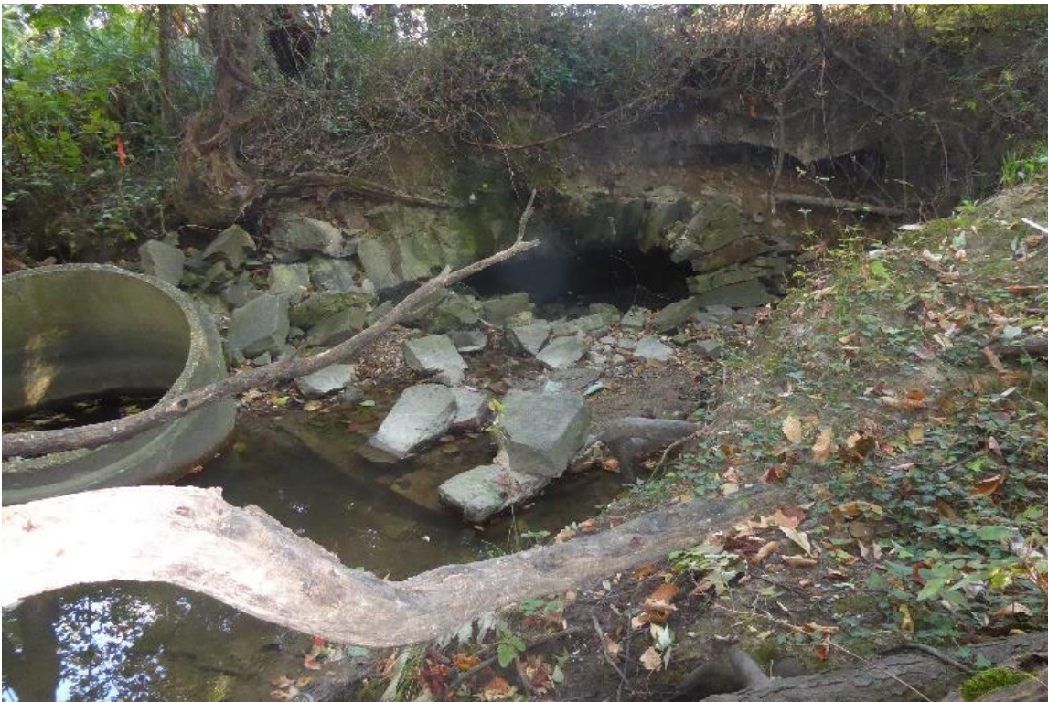
Photo 22. Collapsed Culvert S. of Wilmarco St (10/23/24 [20211])
