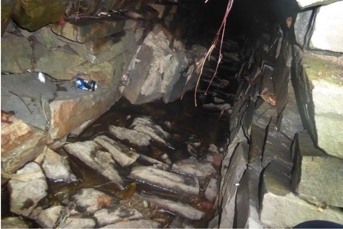
Photo 21. Collapsed Culvert S. of Wilmarco St (10/23/24 [20214])
