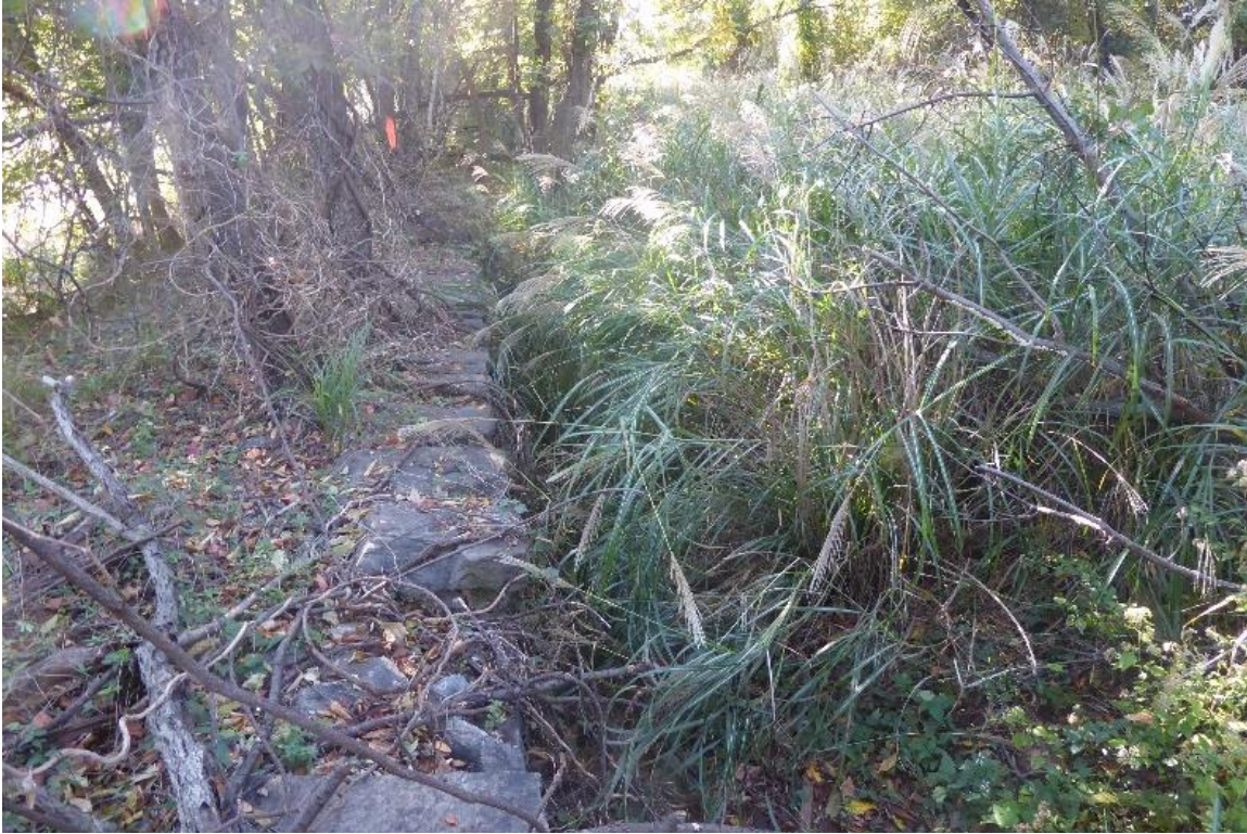
Photo 19. Masonry Wall S. of Wilmarco St (10/23/24 [202018])
