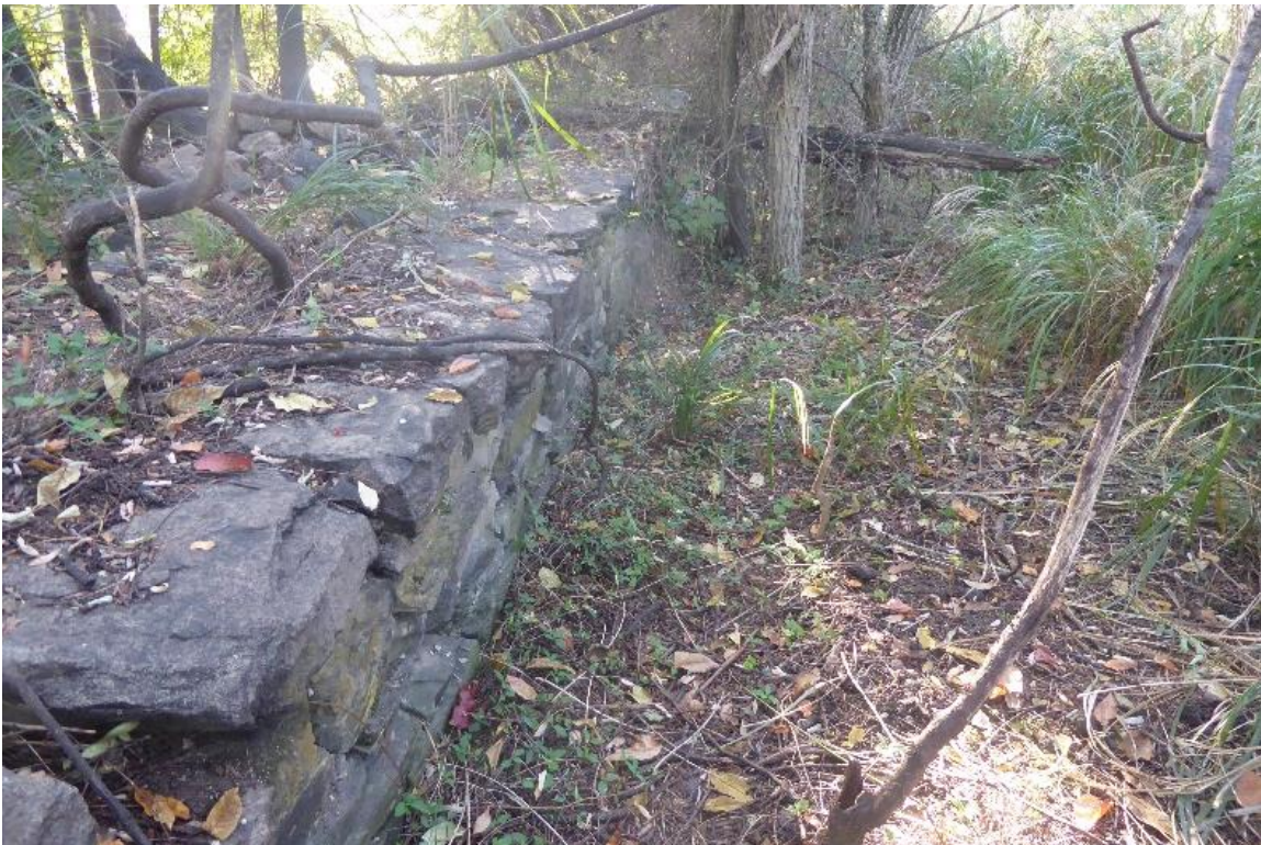
Photo 20. Masonry Wall S. of Wilmarco St (10/23/24 [20208])
