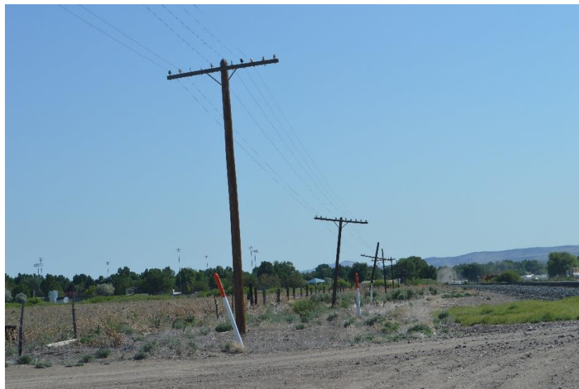
Figure 6. Abandoned overhead utility line near Carlin.
