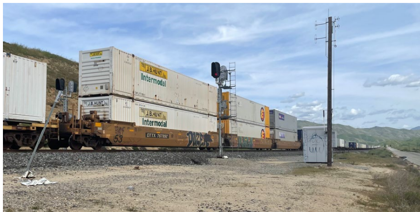
Figure 25: Signal Mast near CP Bena
