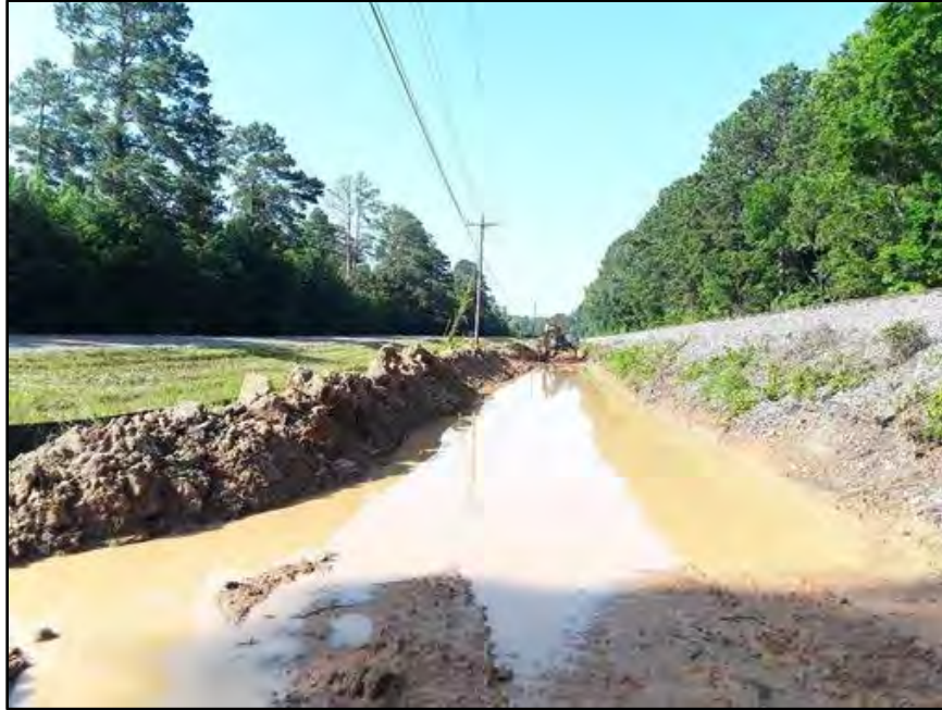
Figure 7. Flooded ROW being drained by a bulldozer; view facing west. (Photograph by D. Holubar June 6, 2023.)
