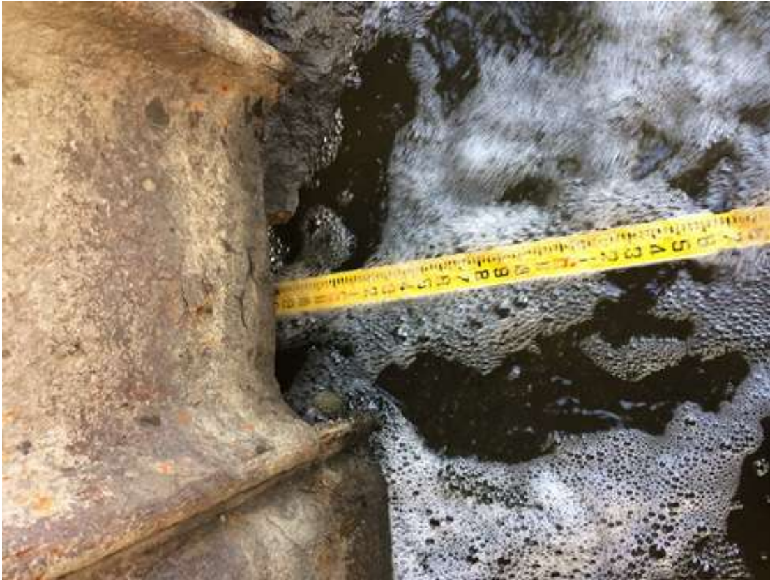
Photo 3 – Tape measure extended 5' beneath footing of Abutment 1.
