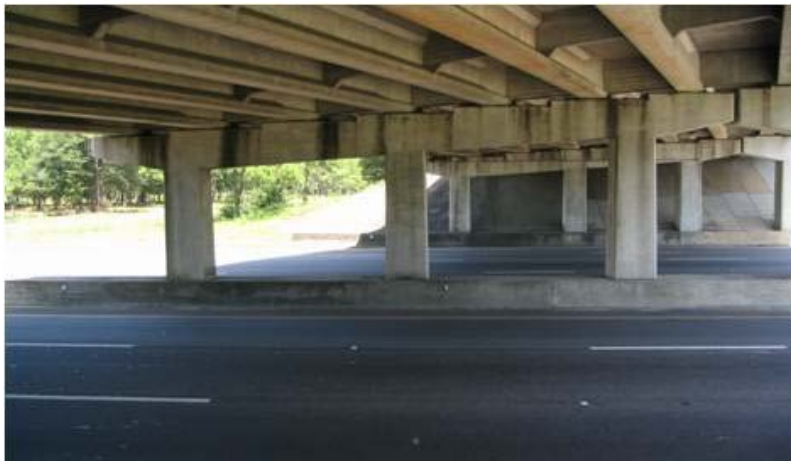
Photo 9: Staining on sides of pier caps
