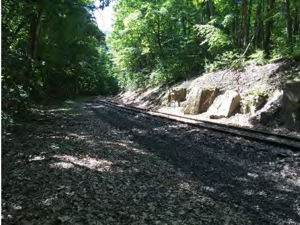
Photo 5. View of the railroad bed as it cuts through bedrock as it extends southeast passed Trailhead 2 on the left.
