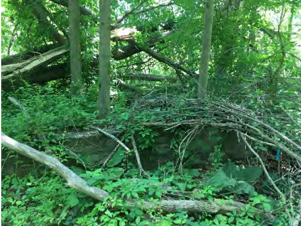
Photo 15. View of the west wall of a concrete foundation that for a smaller building within the depot.
