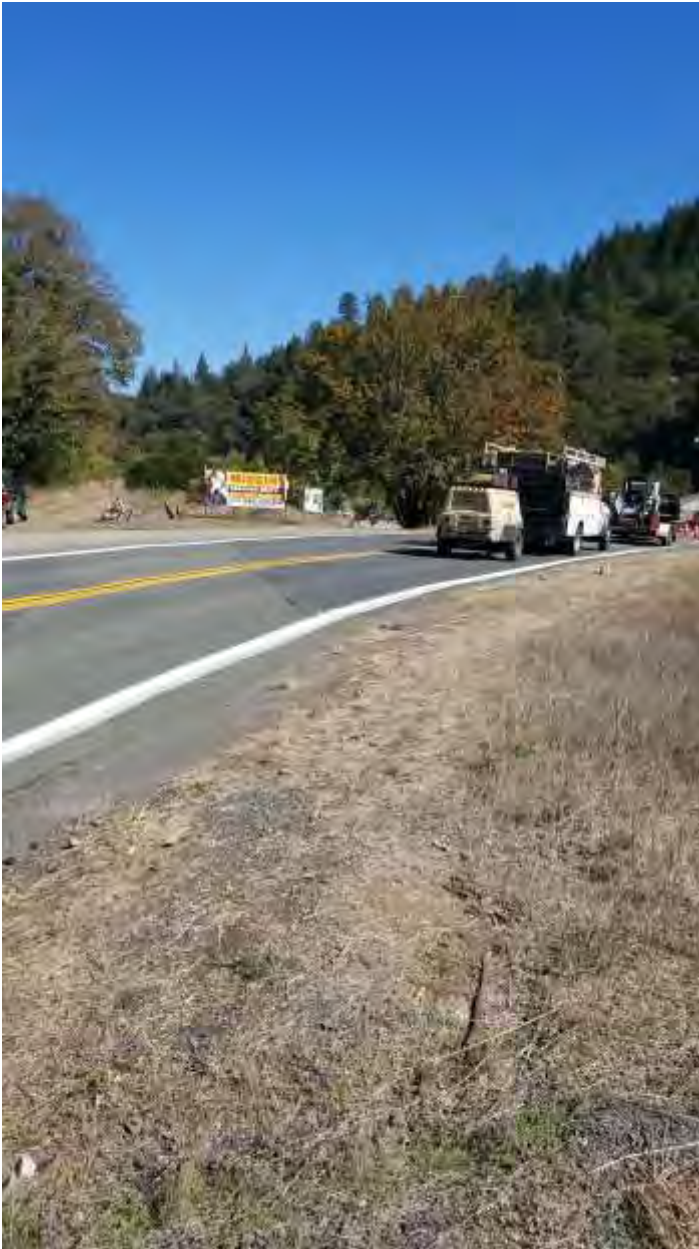
MP 152.2 Covelo road crossing completely removed.
