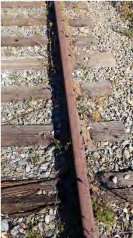
Picture showing tie conditions
