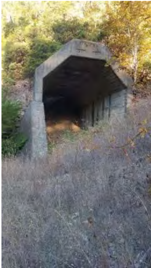
Collapsed tunnel, milepost 145.9 tunnel approximately 400 ft long
