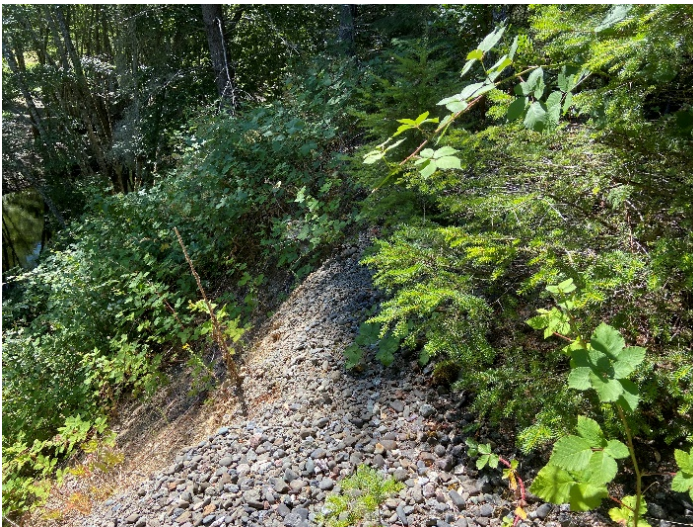
Photo 3 MP 151.6 steep slope at Outlet Creek.
