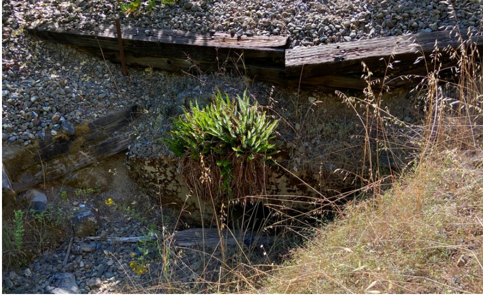
Photo 9 Example of ineffective headwall
