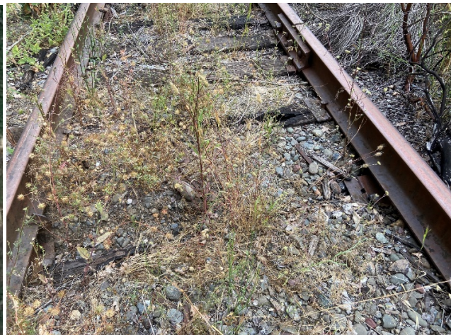
Photo 14 Fire damaged track and substandard ballast.
