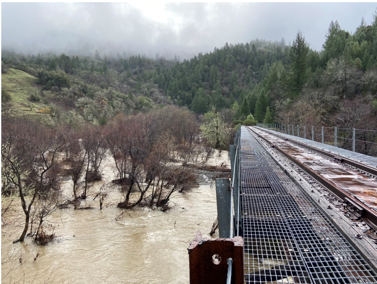
Photo 16 Bridge 151.99 Outlet Creek overflowing banks
