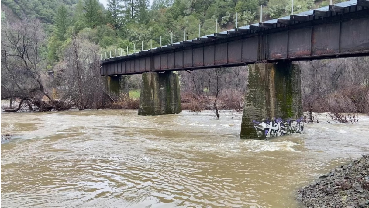
Photo 15 Bridge 151.99 Outlet Creek heavy flow
