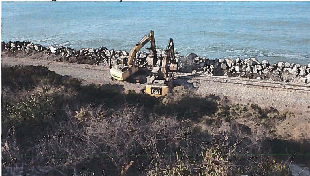
Figure 4. Track Repairs After Erosion in San Clemente
