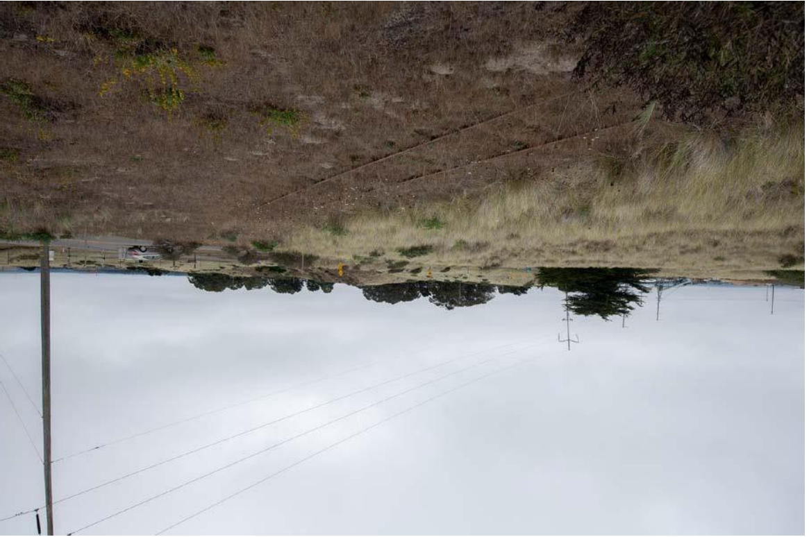
Exhibit N: The state of the remaining rail track on approach to the level grade crossing at approximately milepost 302.0 near Fairhaven, CA.
