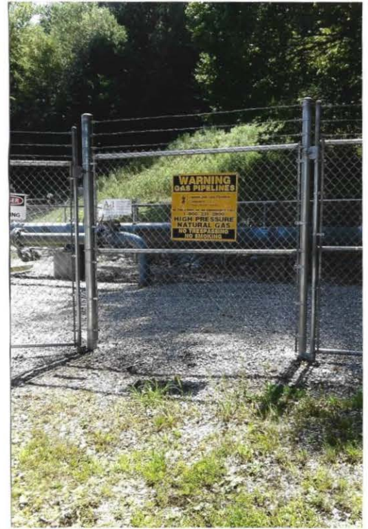
Exhibit C4 Close up of High Pressure Natural gas lines shown on upper level in previous photo
