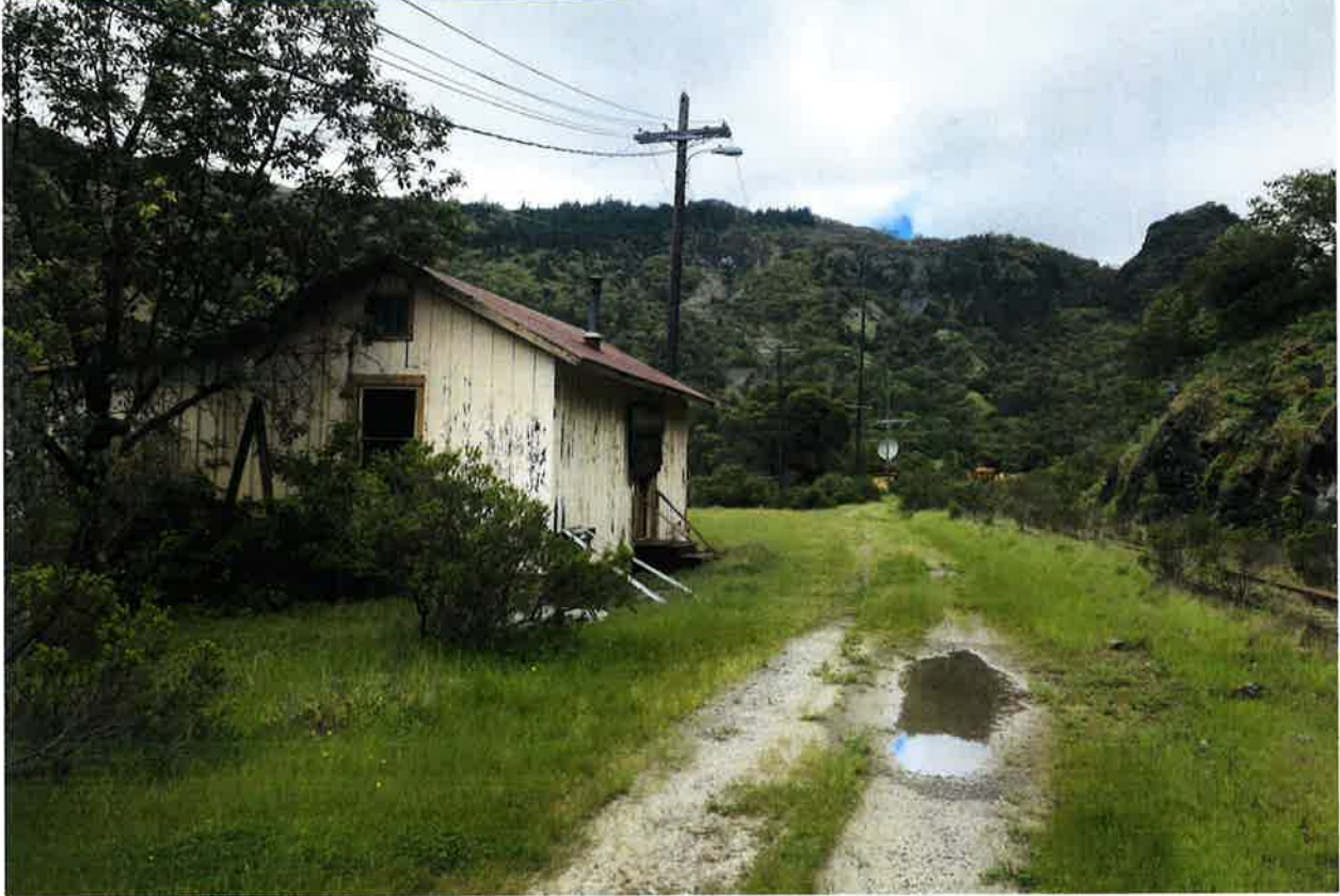
11 Iron Mountain Storage Facility
