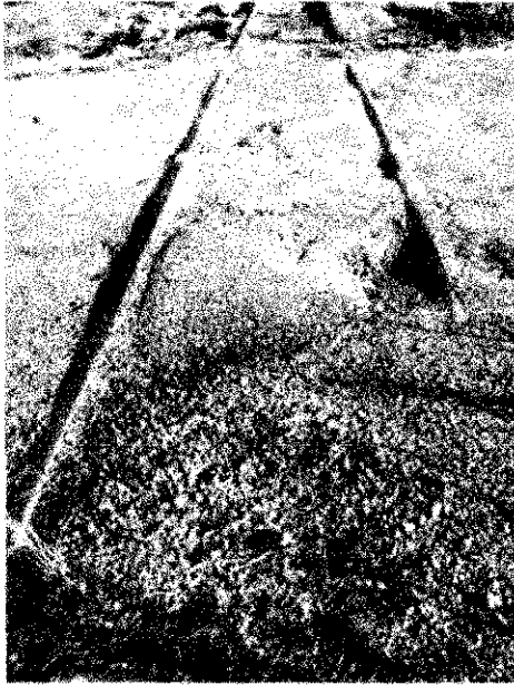
Greenhouse Road Poor asphalt/gravel
