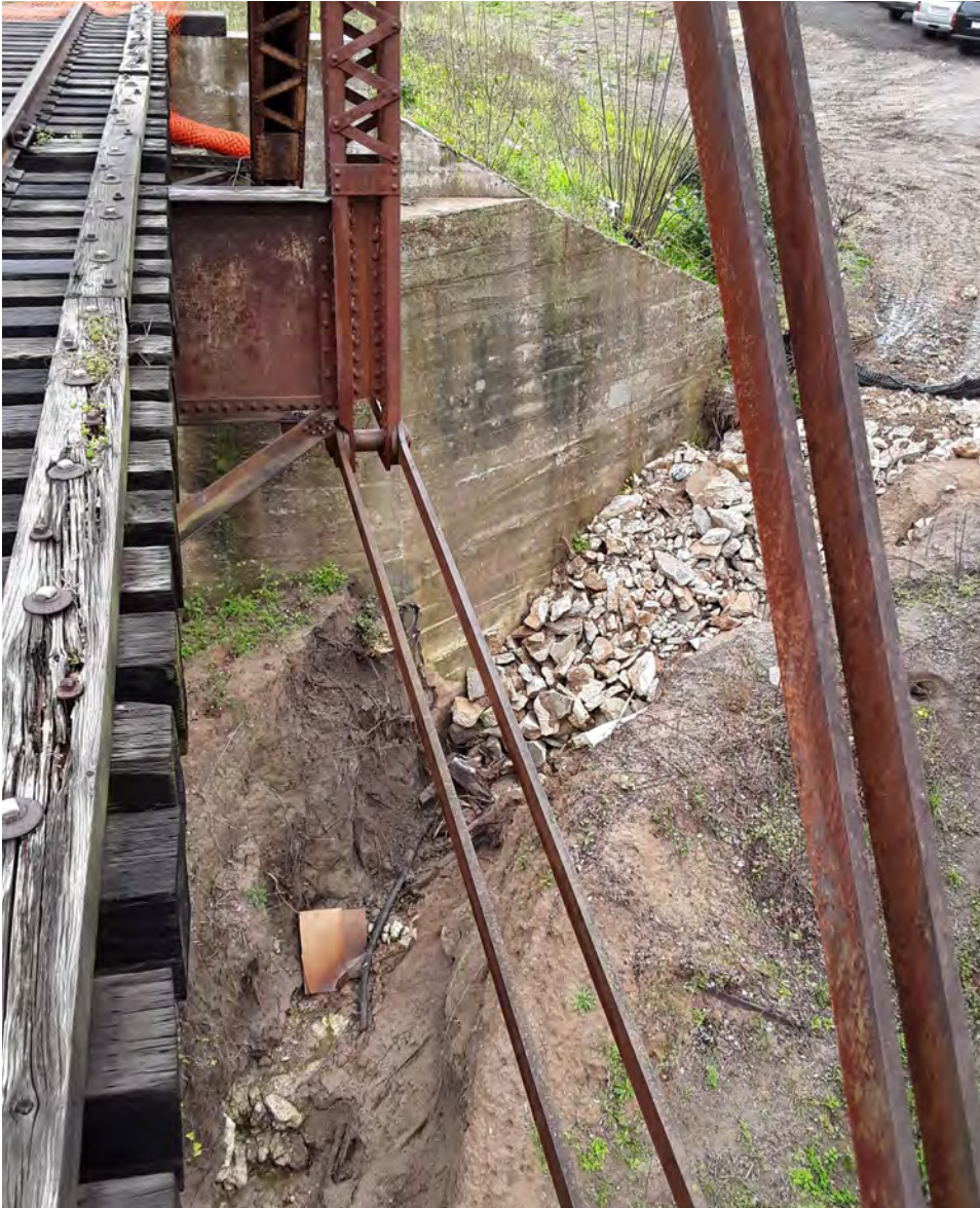
Severe erosion due to storm water runoff from adjacent property; west abutment.
